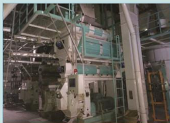
Feed Line after Installation
