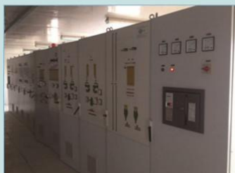
Electric Control Cabinet
