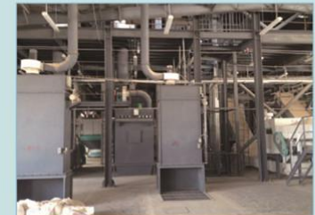
Steel Structure of Feed Line
