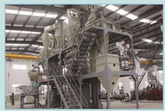
5T/H Feed Line in Bangladesh
