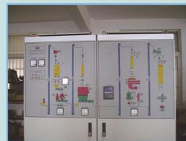
Feed Plant Control Cabinet 饲料生产线控制柜
